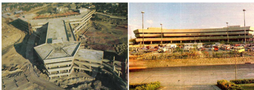
Fig. 7. Locsin's bahay kubo design as applied in the new terminal construction of the Manila International Airport. Left: Construction of the new Manila International Airport terminal that started in 1978. Right: Completed structure of the Manila International Airport.
