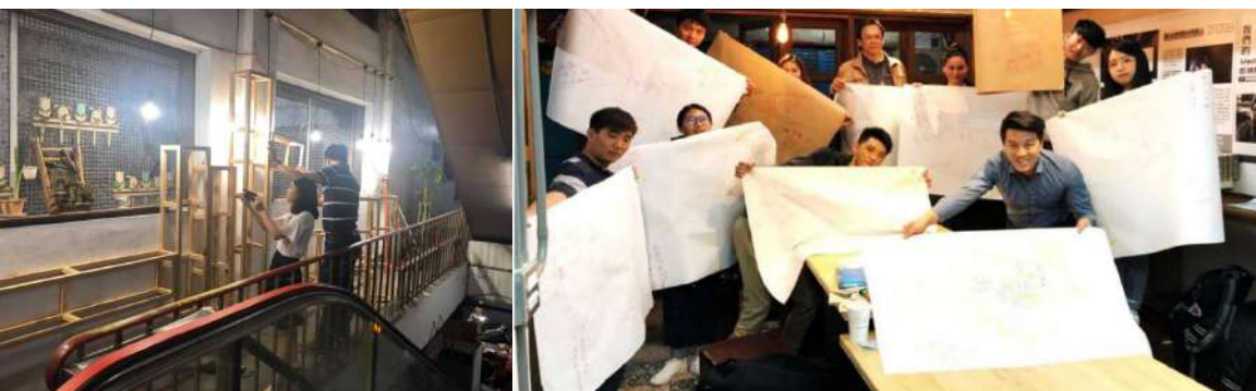
Fig. 7. Chung Hua University – Department of Architecture and Urban Planning master’s students during planning in the actual site (Dongmen Market’s third floor), bachelor’s students renovating and enlightening the escalator
