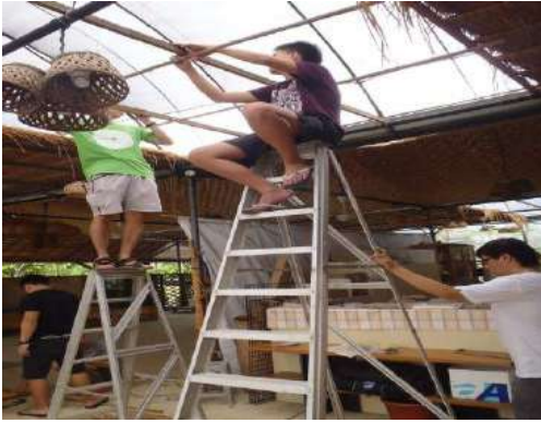
Fig. 5. Volunteers installing lighting shades made out of baskets in SLK's Living Room
